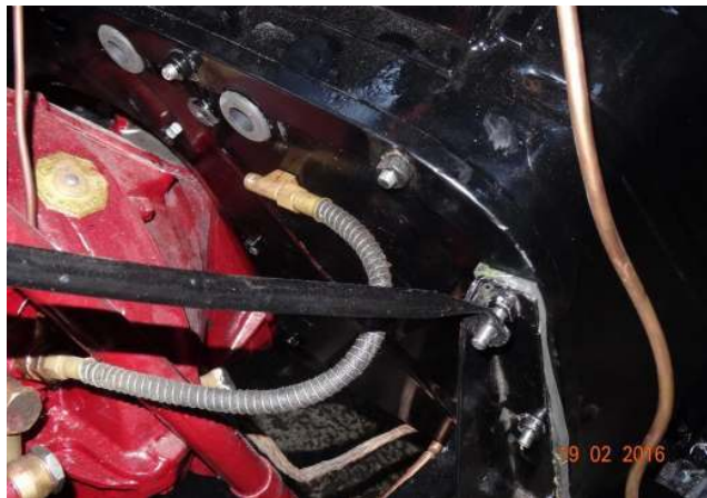
The two cable grommets, the oil gauge brass adaptor fixed to the bulkhead and I know the rad supports need the nuts fitting.
