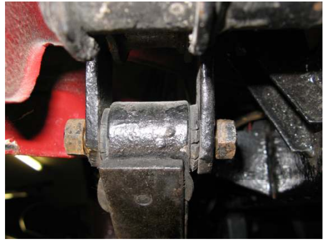
Photo 2 illustrating the limited space in which to work due to the proximity of the rear wing trailing edge to the spring hanger. Also visible is the wear on the rubber bushes in the spring 'eye' and a spring interleaf pad with its 'dowel' located in the spring leaf.
