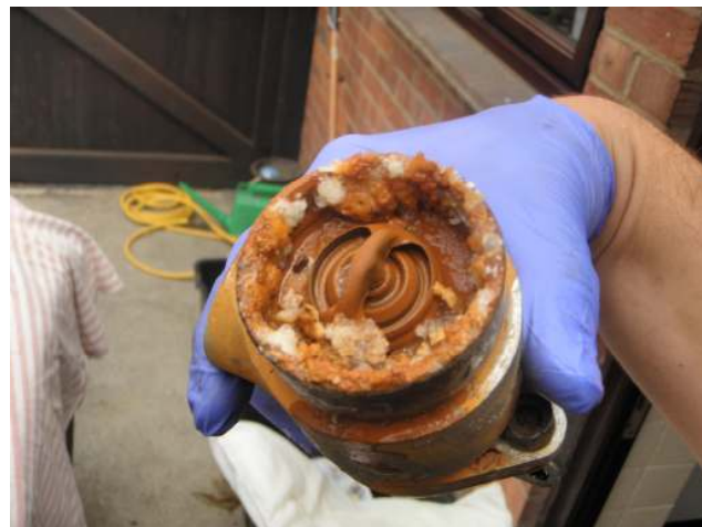
Photo 1 showing the ‘horrible crud on the new thermostat which had only recently been fitted.
